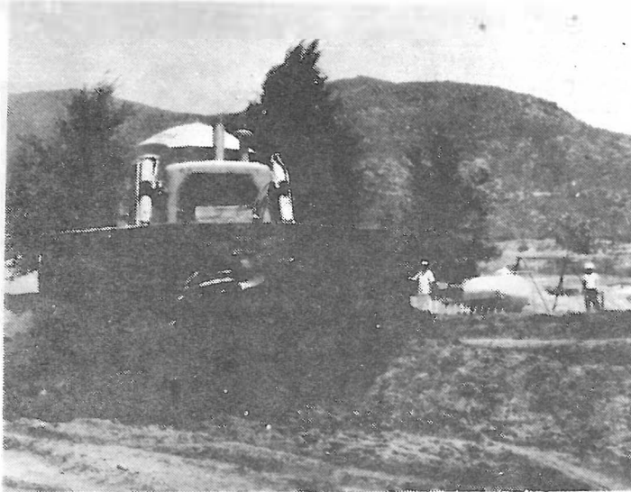
Here is big dozer pushing tons of earth to make fill for new Baptist Church of the Willows. On preceding page photo shows Paul Thorp, left, with hose sprinkling, with Robt. Bostrom at right. Boy is Otto Hirr, 8, son of the Bostrom's daughter Olive, of Pt. Loma.
